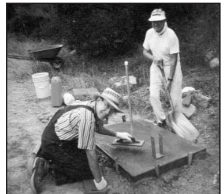
Volunteers John Broesamle and John Melville pour concrete and install Mutt Mitt dispensers at sites in the Ojai Meadows Preserve and on Shelf Road.
