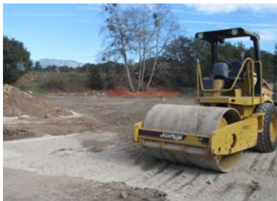
Above: Compacting road base on new horse trailer and staging area at new trailhead with Topa Topa bluffs in far background.
